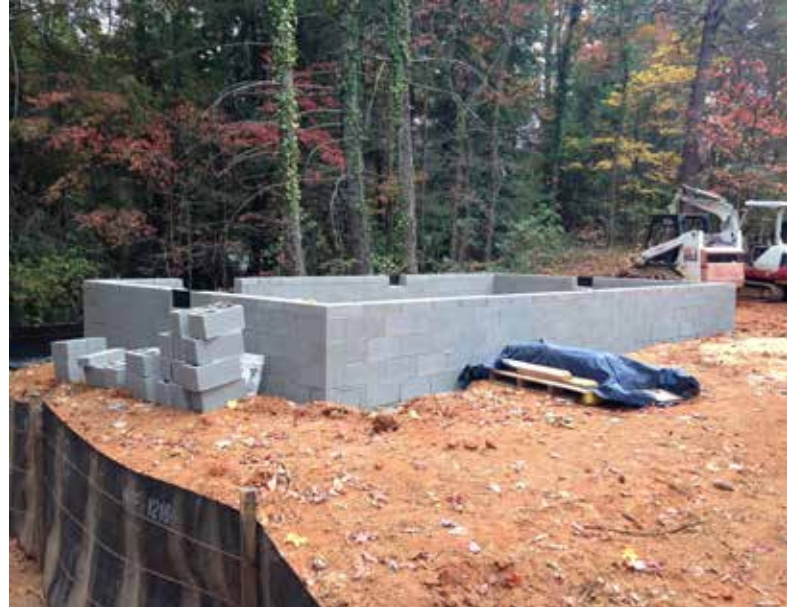
Construction is under way for the first of two "bunkhouses" at the LES Center.
